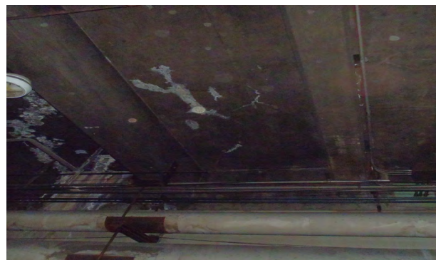
FIGURE 8: WATER DAMAGE IN SOUTH TUNNEL
