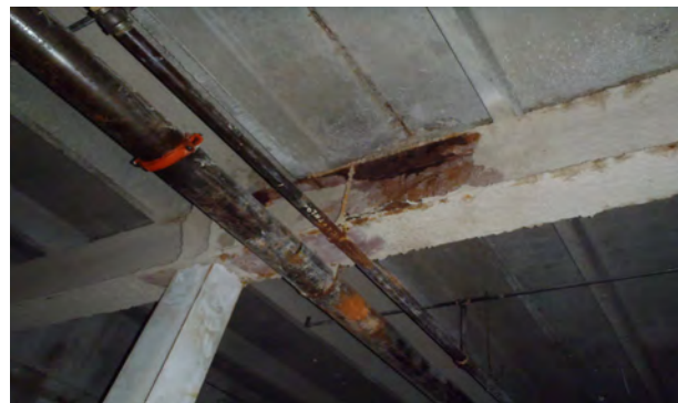
FIGURE 7: CORRODED STEEL UNDER FIRST FLOOR
