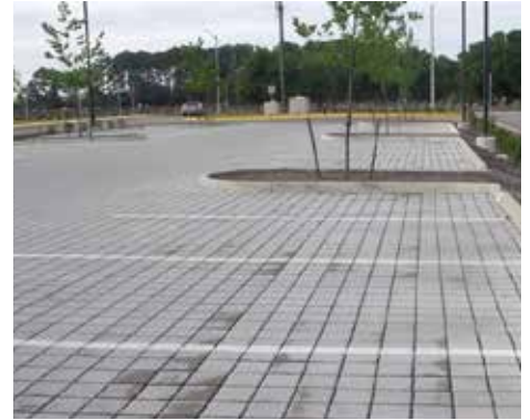
Parking lots built with permeable pavers reduces the runoff that enters the stormwater system.
