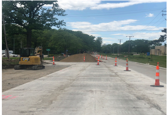
Work continues on the reconstruction of Civic Center Drive between Northwestern Highway and Lahser.
