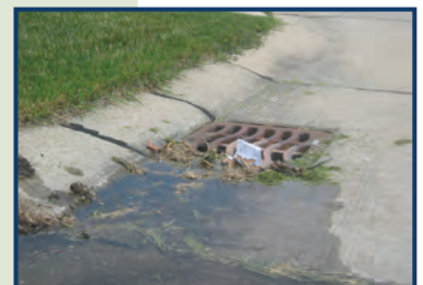
Keep storm drains clear of debris to reduce pollution entering our lakes and rivers.
