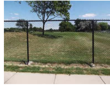
Photo 2, Vinyl Coated Chain Link
